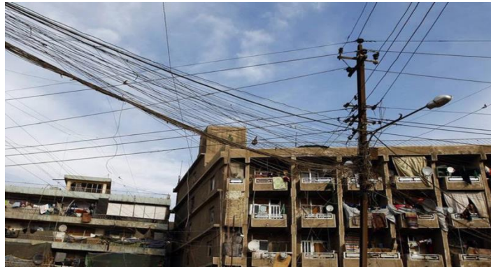
Figure (1): Random distribution of electrical generator wires.
