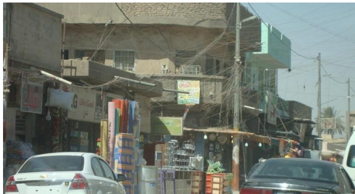
Figure (2): Random distribution of electrical generator wires and significance for places.
